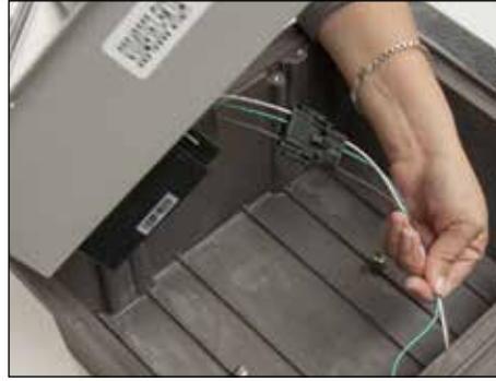
8. Begin installation of LED upgrade by connecting electronic driver wiring to line voltage
