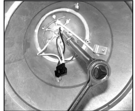
Junction Box (By Others)
