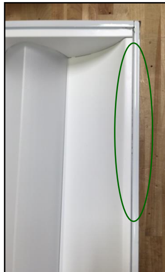
Figure 8. No gap between door frame and side of housing.
