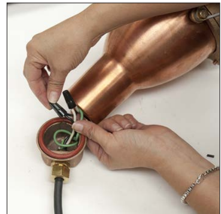
NOTE: On the C54, make a connection from LED optic assembly to existing cable using connectors by others.
